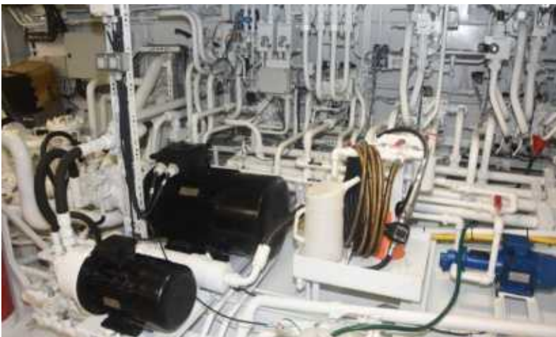
The array of pipework across the aft end of the engine room.
