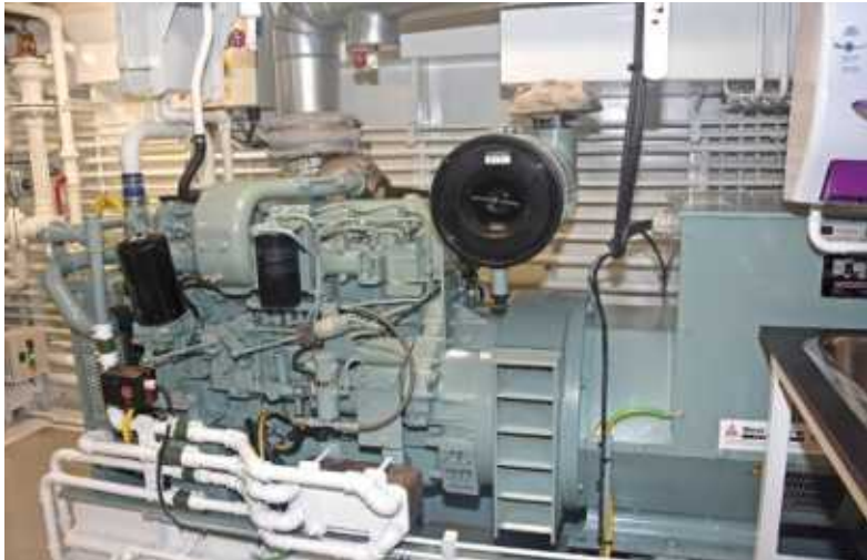
One of two Mitsubishi 6D16 auxiliary engines that drive 116kVA Newage Stamford 415/3/50 generators.
