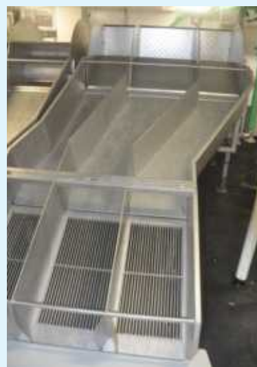
Pivoting chutes connect the fish washer and gutting machine to selection hoppers in the fishroom via deck coamings.
